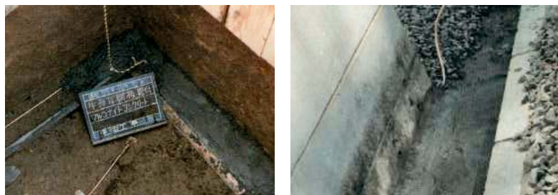
Laying SAN-EARTH M1C *One 25kg bag of M1C will cover approx. 3 meters (width 30cm)
