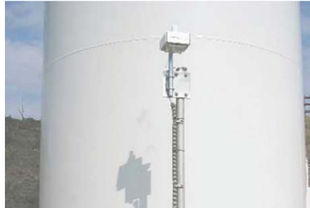
Installed on the side of a wind turbine
