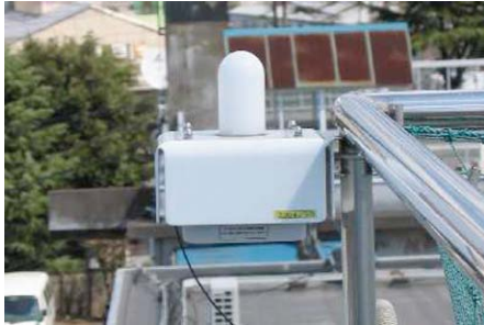
Installed on the fence of a building roof
