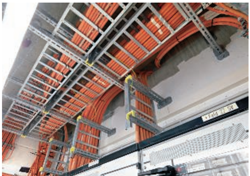
Function maintenance system in the power supply centre
